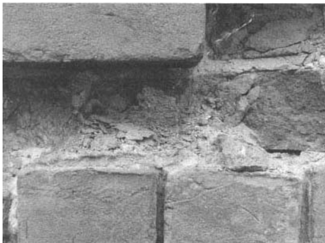
Fig. 76. Freeze-thaw processes have caused these construction bricks in Ouray, Colorado, to exfoliate.
